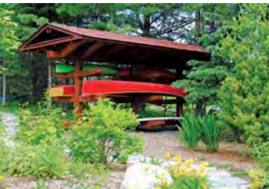
A custom canoe shelter was built along the granite path, making it easy for the homeowners to access canoes and paddleboards on their way down to the lake.
